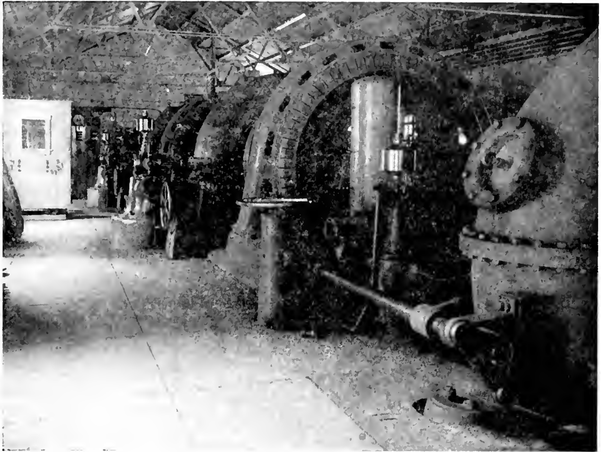
Interior of Tygh Valley Generating Station - July, 1910.
